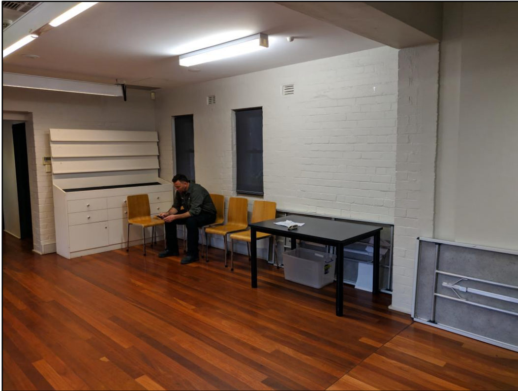
Figure 8: Existing painted brick walls and timber framing will be retained. Modern cabinetry and skirting containing wires will be removed.
